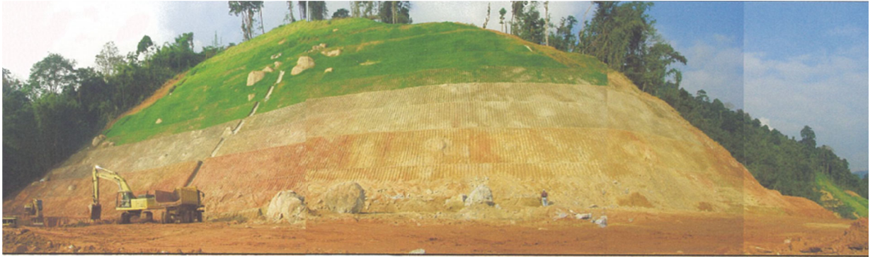
Fig 3A: This cut slope has no large upslope catchments for excessive infiltration. No sign of seepage, no severe geological discontinuities except some localized boulders. Hence, with proper slope protection & slope drainage the risk of excessive infiltration is practically negligible or the slope is bound to be safe and stable. Some block sample samples from distinct layers should be taken for CIU tests for quantitative stability analysis to ascertain the local & global stability. With regular routine inspection and maintenance by suitably qualified personnel as per recommendations by JKR Guidelines on Slope Maintenance in Malaysia (Aug 2006) and some simple instrumentation monitoring, the slope should be reliably able to ensure long safety and stability.
